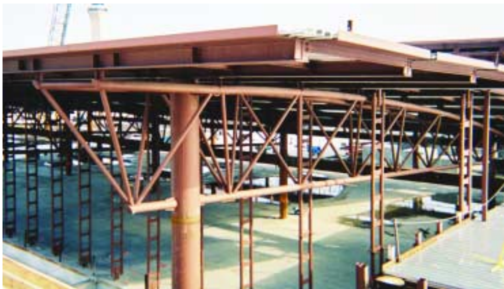
Above: Details of the HSS connections for the tri-chord trusses in the INS Hall. (Details courtesy Walter P. Moore.)
